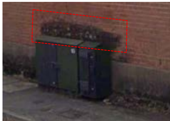
figure 149: Telecommunications cabinet – Lower Street
