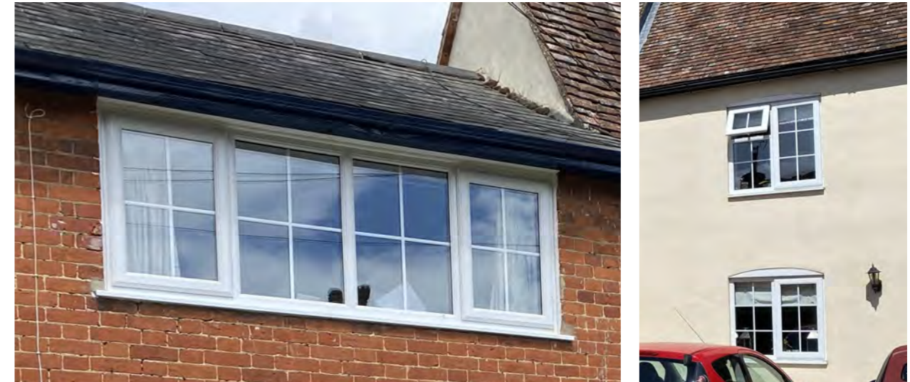
Figure 239-240: Examples of poorly detailed modern replacement windows. Flush to the surrounding walls instead of recessed, applied or 'stuck on' glazing bars' heavy opening casements overlapping 'storm window' style instead of flush with the surrounding frames, material uPVC.
